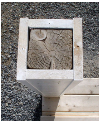
Fig. 7 This wrapped stair-post shows how the twisted 4x4 has been squared up.
